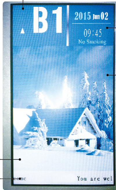
Real-time Elevator Status Display
